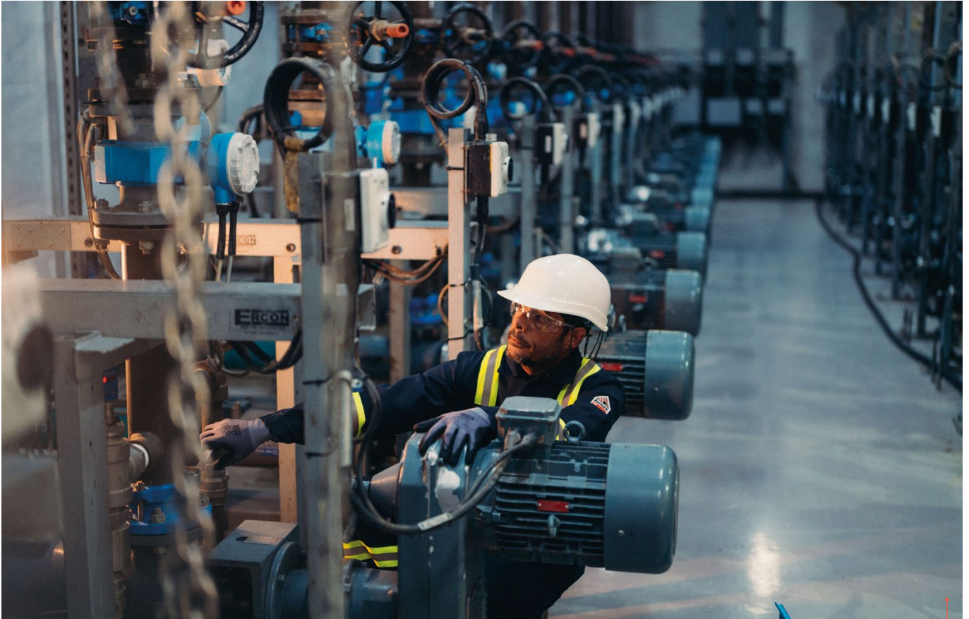
As Samra wastewater treatment plant, Jordan. This plant treats and redistributes wastewater from the capital and the surrounding area. 25% of the country's agricultural water requirements and 12% of global water needs (for domestic use in particular) come from this site.
