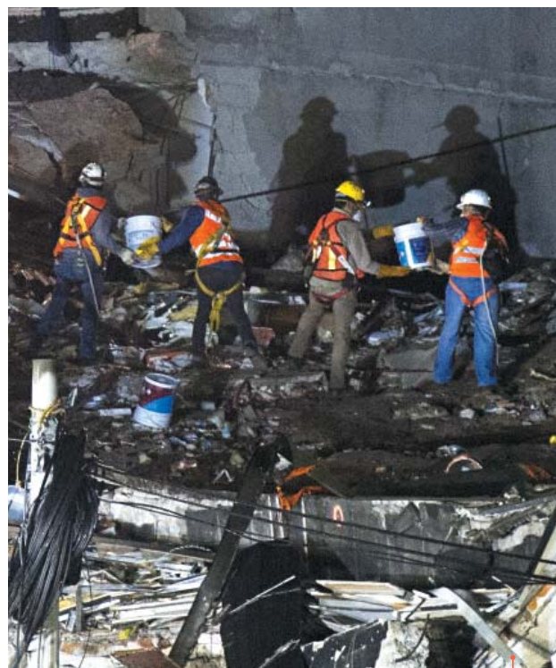
Mexico, September 25, 2017. Rescue work in a collapsed building
