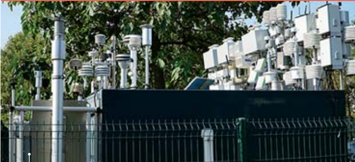
Installation of microsensors as part of the AIRLAB Micro-Capteurs 2019 Challenge ©MTES (Ministry for the Ecological and Inclusive Transition)
