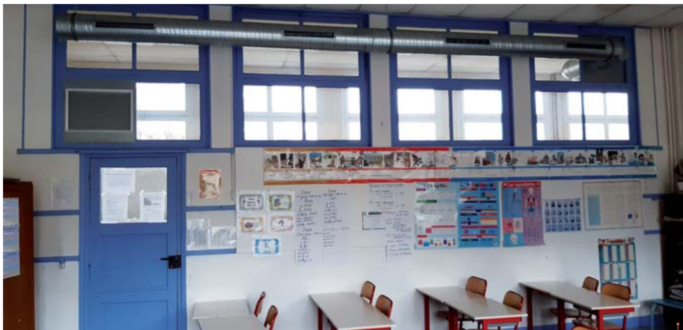
Semi-centralised dual-flow air handling unit, La Fontaine elementary school (Le Raincy, France), class number 3 - © Jade Lachery
