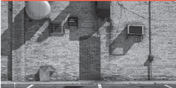
Ventilation units on a building façade
