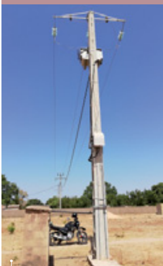
Junction point between the Sénélec medium voltage grid and the low voltage network operated by NSRESIF, village of Diaglé
