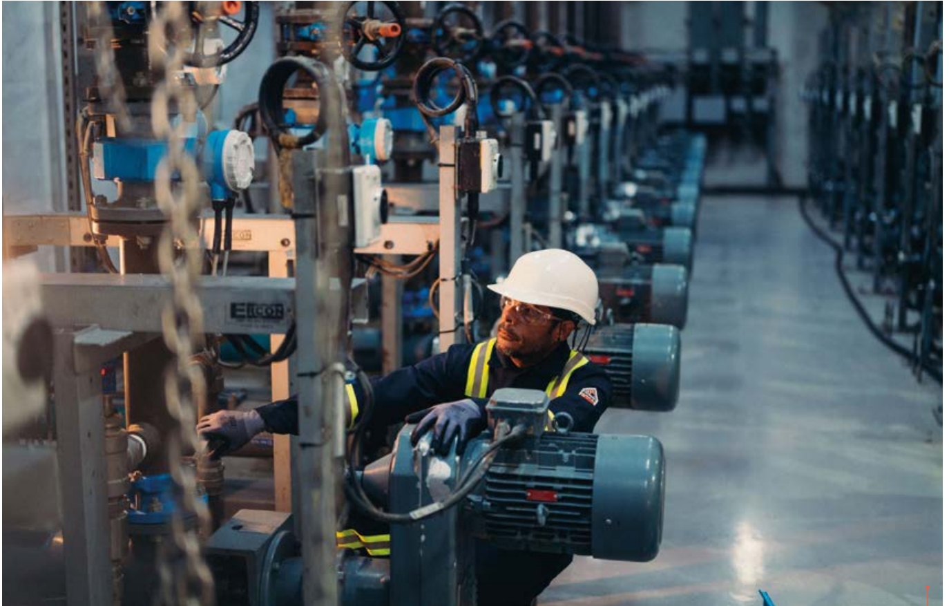
As Samra wastewater treatment plant, Jordan. This plant treats and redistributes wastewater from the capital and the surrounding area. 25% of the country's agricultural water requirements and 12% of global water needs (for domestic use in particular) come from this site.
