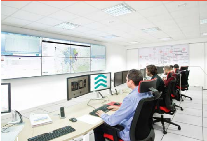
Vig'ileo, Veolia's latest hypervision center for managing the water service of the future - launched by the Métropole Européenne de Lille.
