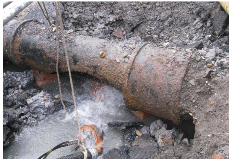
Corroded water pipe
